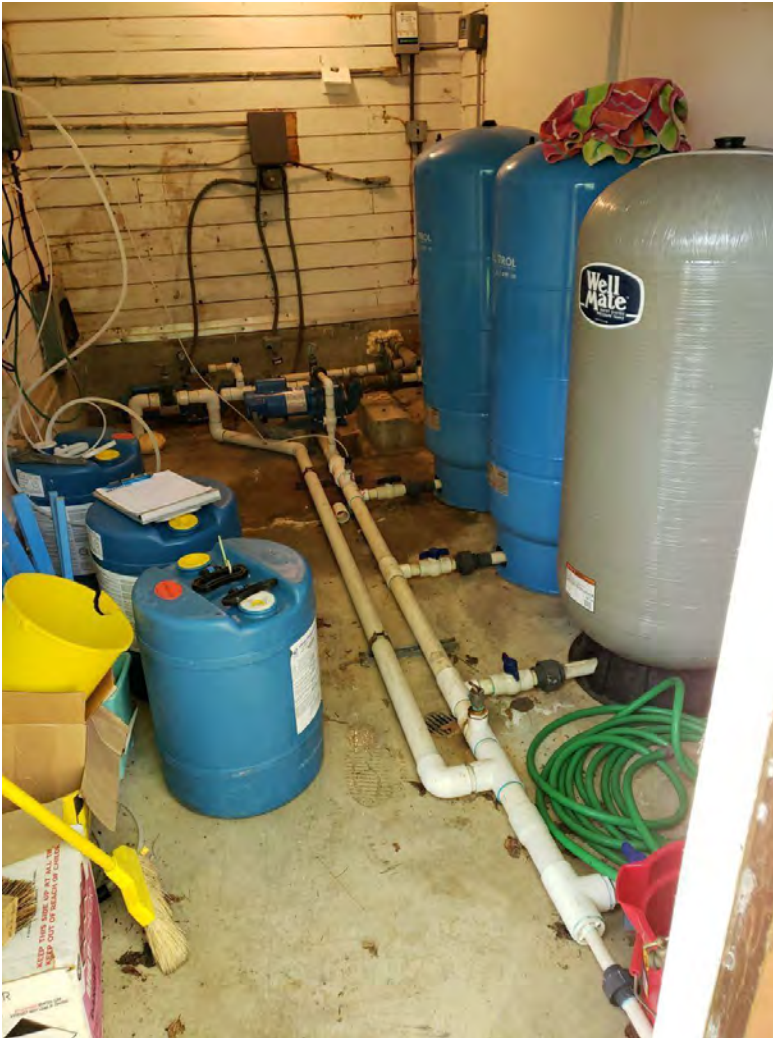
Figure 3: Well pump house interior
